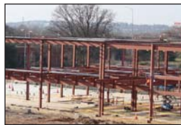
Over winter break, MJ Harris Construction made advancements on the framework of the Football Operations Center.
