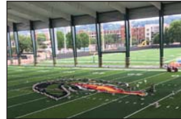
On June 1, MJ Harris put the finishing touches on the second turf field under Legacy Pavilion with adding the Blaze Head logo at the 50-yard line.
