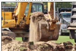
Construction officially began on September 19 when Bulldozers started digging into the ground for the Football Operations Center.
