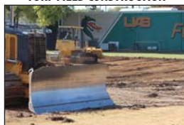
Construction on the first of two turf practice fields begins. Once completely finished, the entire facility will have two turf fields and one grass field.
